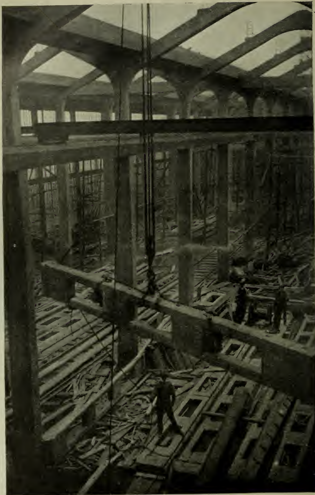
NEW WORKSHOPS FOR THE GAS LIGHT & COKE CO.: HOISTING PRE-CAST CONCRETE PURLINS INTO POSITION.
